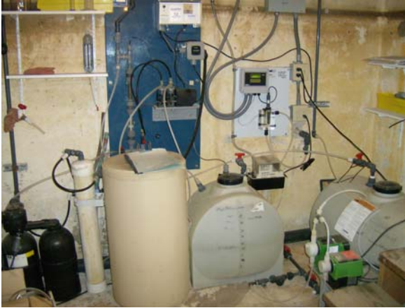
Vosburg Delores Tunnel Chlorinator
