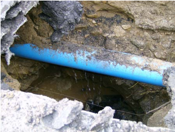
Pasadena Glen Water Main Break
