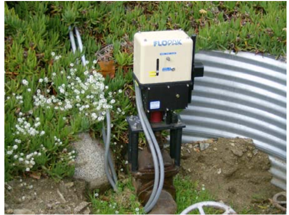
Vosburg Reservoir Flo-Loc Valve
