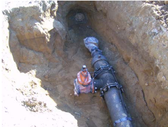
Valve for New Fire Hydrant
